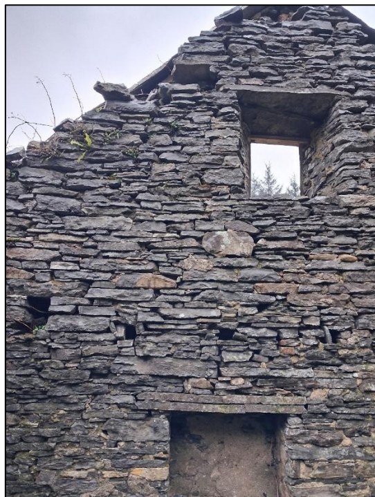
Plate 3-41 Derelict stone building classified as Stone walls and other stonework (BL1).
